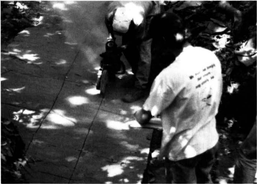
Figure 1. Using a cut-off saw, sections of the trackway were cut along a marked grid and were removed and taken to the museum to be studied.
